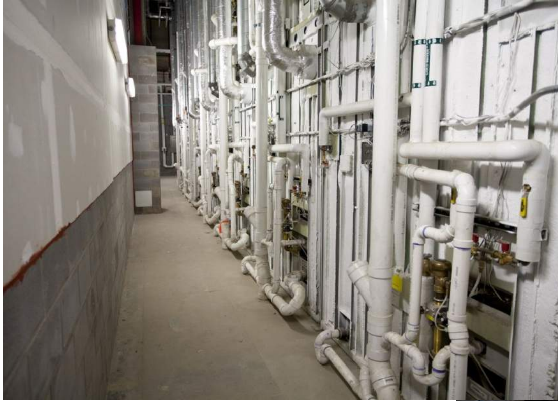
Allegan County Jail – Rear Mechanical/Plumbing Chase
